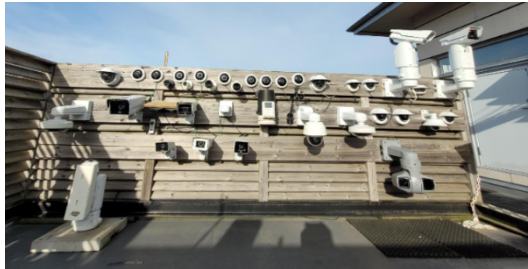
Figure 7. Axis test cameras installed on site in Lund.
